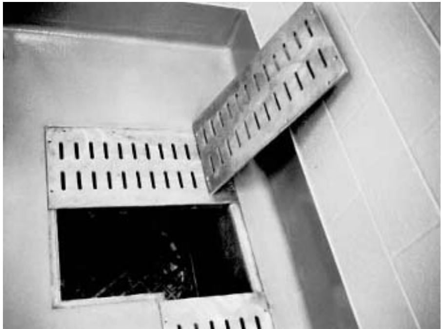
► Trench drain in remote corner. Animal Facility, Clemson University, Clemson, South Carolina. GMK, architect.
