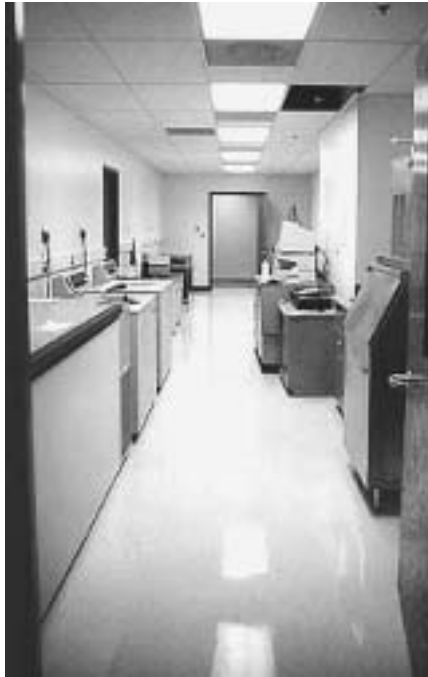
◀◀ Shared deionized water and ice machine on each floor. Stevenson Center Complex Chemistry Building, Vanderbilt University, Nashville, Tennessee. Payette Associates, Inc., architect.
