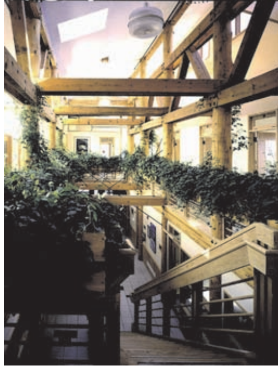
Figure 3-23. A graywater system provides water for interior planters in the French Wing.
