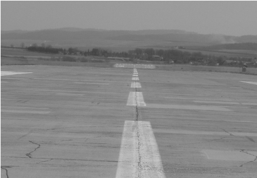
Figure 4-16 One-sided transverse runway slope and changes of longitudinal slopes are clearly visible (Photo: A. Kazda)
