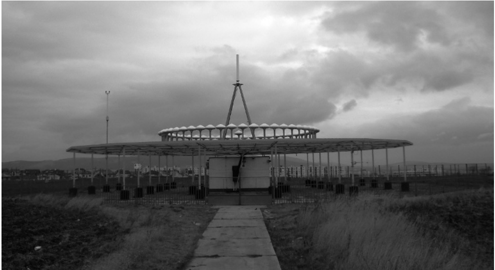
Figure 17-6 D-VOR/DME ground station Nitra
