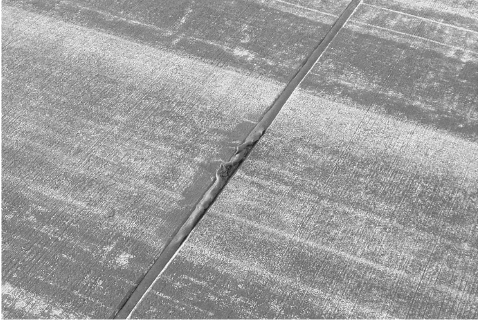
Figure 8-4 Damaged sealing compound on a joint (Photo A. Kazda)
