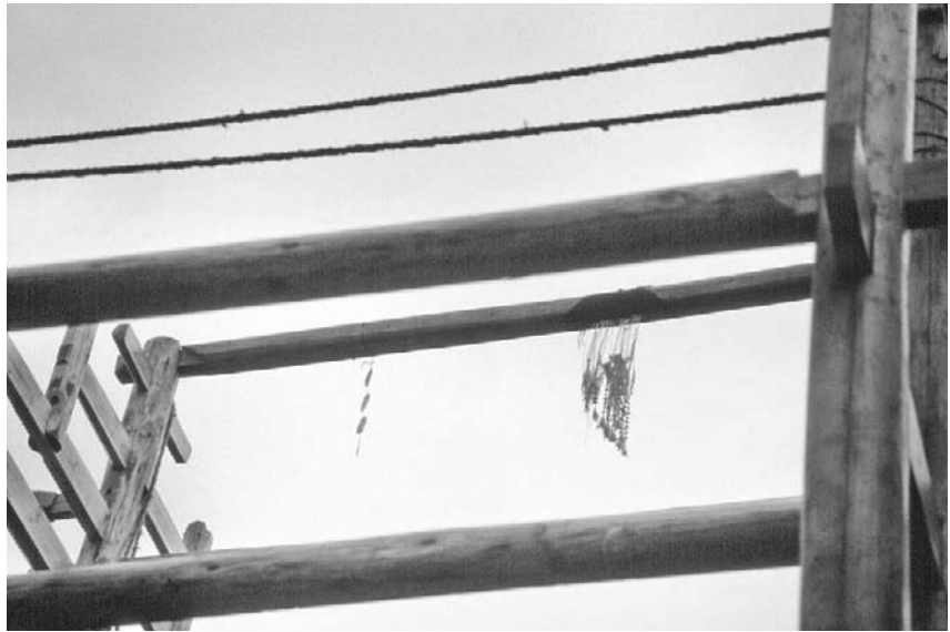
Figure 4.30 The main roof ridgepole of a Dong house in Pingyan village, Sanjiang region, Guangxi province, showing the colorful feather-flowers tied to the ridgepole at the building ritual. Source: Photograph by Xing Ruan, 1993.
