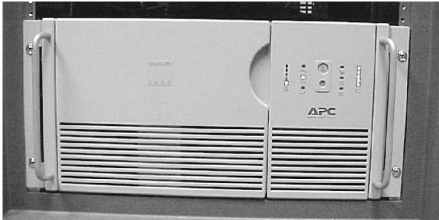
Figure 14-13. A rack mounted UPS used for network servers
