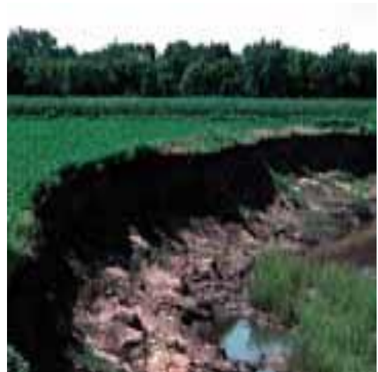
(Erosion by Floodwater)
