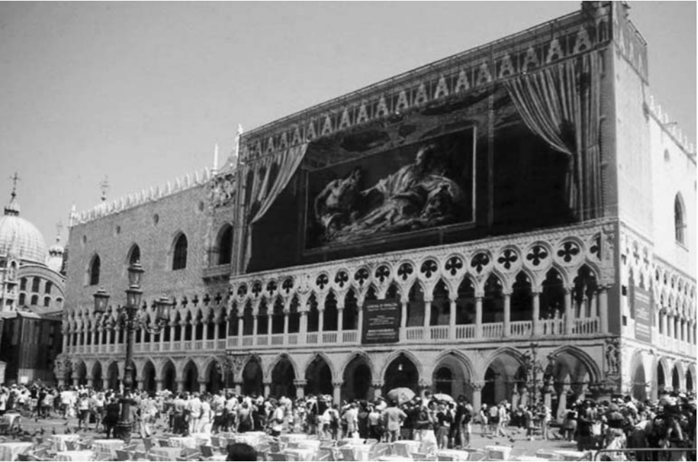
Figure 34.5 Doge's Palace, Saint Mark's Square in Venice. Source: Gary Hack. Note: A construction shroud that "peeled back" the façade to expose the paintings within provided a new vision for St Mark's Square, Venice, during the multi-year renovation of the Doge's Palace.
