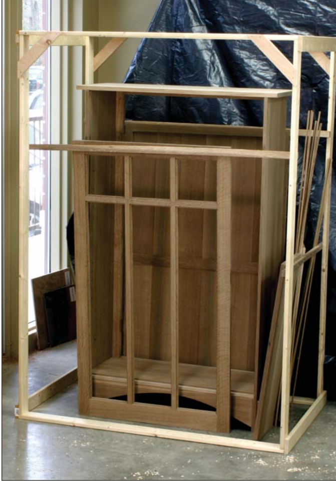
After "fuming" for 24 hours the tent was aired out and the plastic removed. Here you can see the construction of the tent frame, and the change in color.
