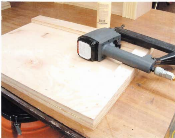
15 Cut buildup strips to fit the base cabinet tops and glue and staple (or screw) them to the underside of the tops. Plane or sand the edges of the buildup strips flush to the edges of the tops.
