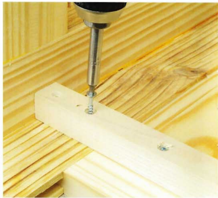
10 Using glue and screws, install the bottom front, back and side cleats.
