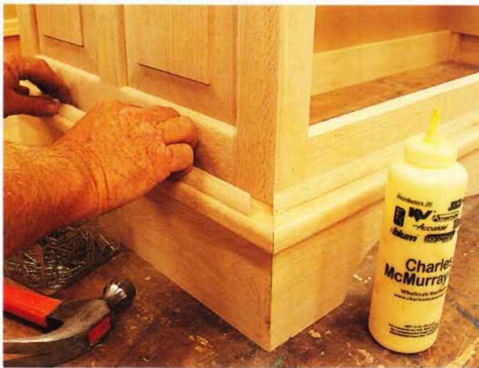
5 Cut the front and side base quarter-round moulding to fit. Glue and nail.
