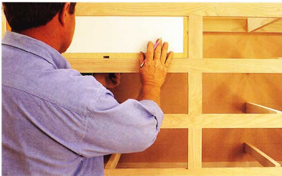
7 Install the drawer guides using an assembled drawer to center the drawer guides. Align the guides horizontally with the lines on the 1/4" back panel.
