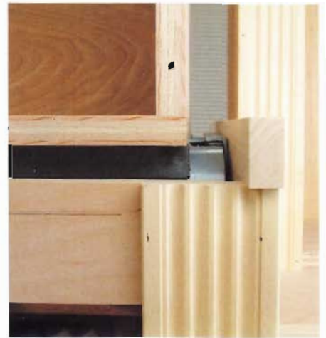
23 Assemble the TV lift box, install it on the TV lift and raise the lift to its fully elevated position. Double-check all measurements for the top of the center cabinet. One of the side strips for the top has been placed on the top of the center cabinet to show the relationship of the edge trim to the TV lift box. The top of the bottom panel of the TV lift box will be flush with the top of the cabinet.
