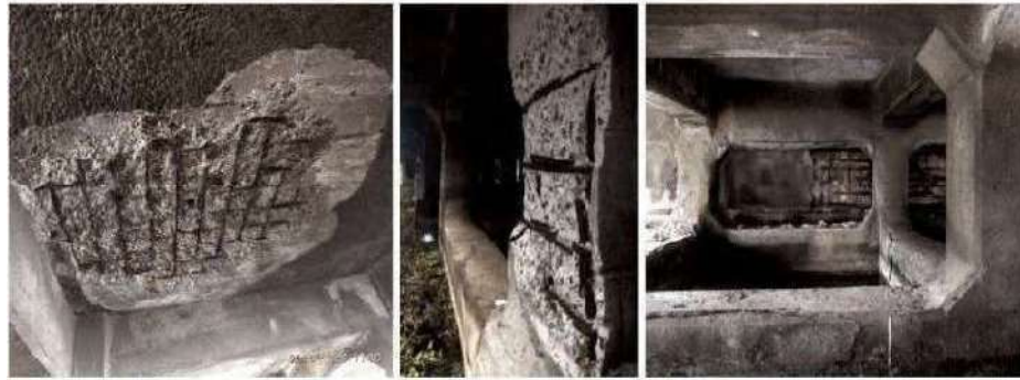
Figure 2.25: Exposed Rebar in Deck Slab, Piers and RC Fenders
