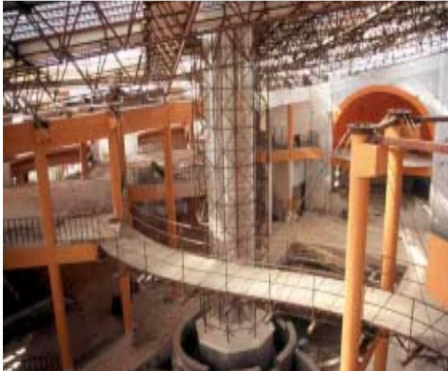
An inside view of the PEDA Bhavan in Sector 33, Chandigarh. A Tribune photograph
