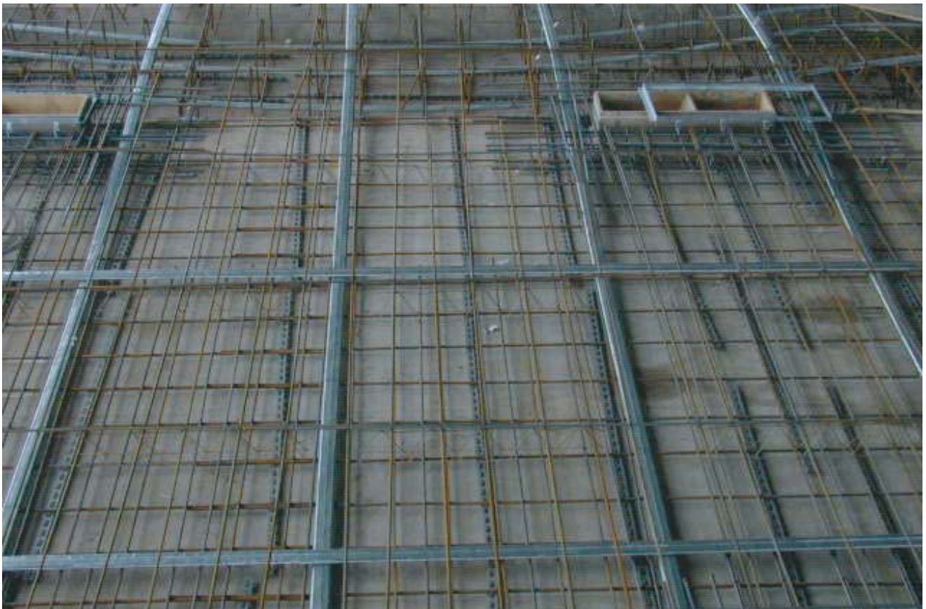
Figure 7.33 Slab and beam tendons in post tensioned slab (courtesy of Sir Robert McAlpine Ltd)
