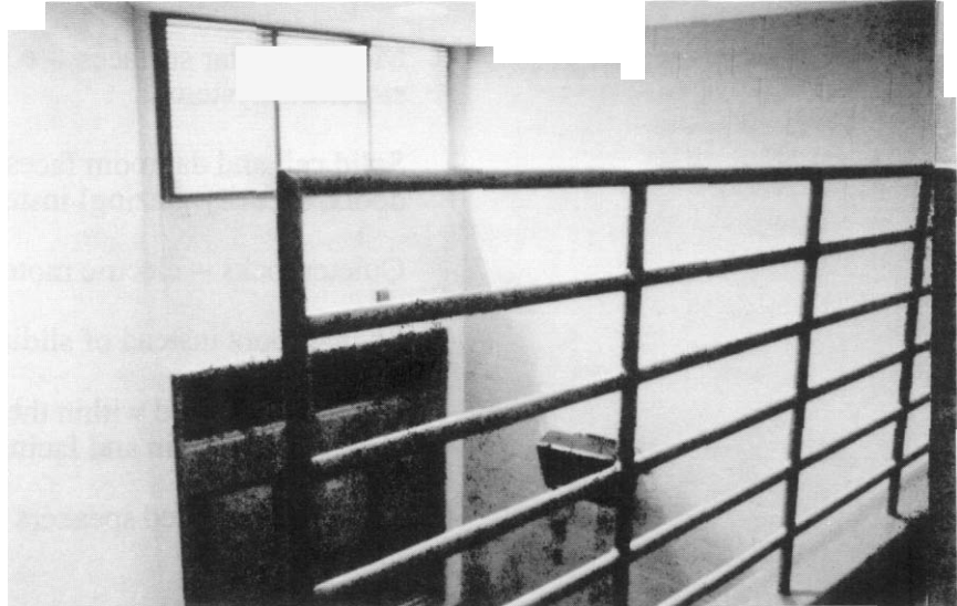
Dayroom clerestory shining toward cells (on right) and not toward the officer's vantage point.
