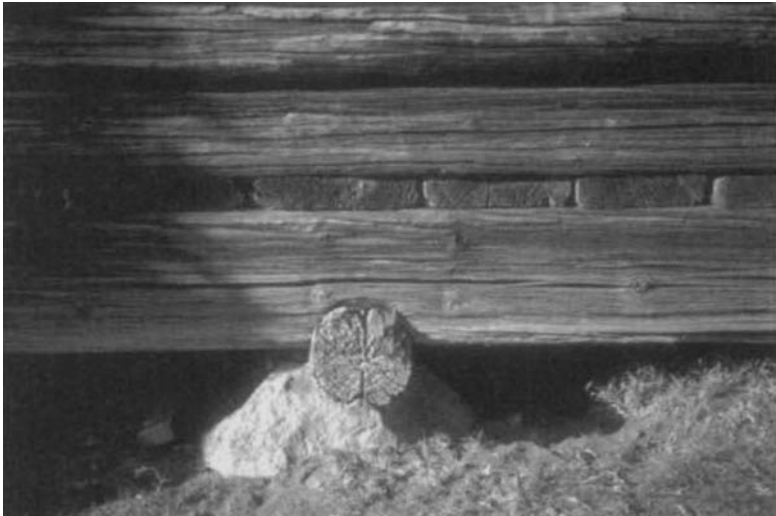
Raising the floor from the ground isolates inhabitants from the cold and damp of the earth. Photograph by Simon Beason.
