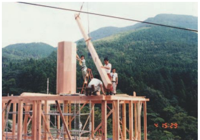
▲ 8.18 The RF beams are positioned on the temporary prop. (Photo: Yoichi Kan.)
