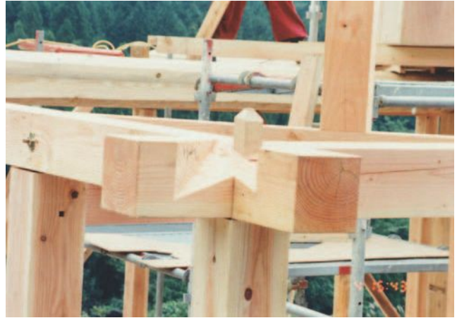
▲ 8.16 Traditional Japanese timber joints are used throughout the building. (Photo: Yoichi Kan.)
