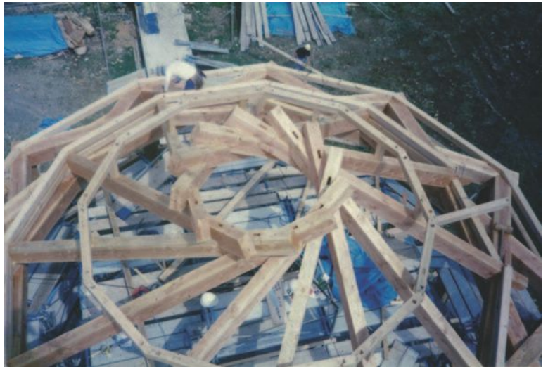
▲ 7.42 The structure of the RF roof is in place. (Photo: Kazuhiro Ishii.)
