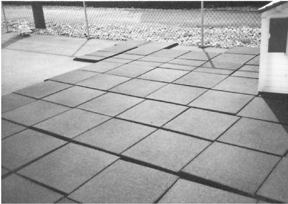
Figure 4.34 Photograph of improperly installed playground surface pads.
