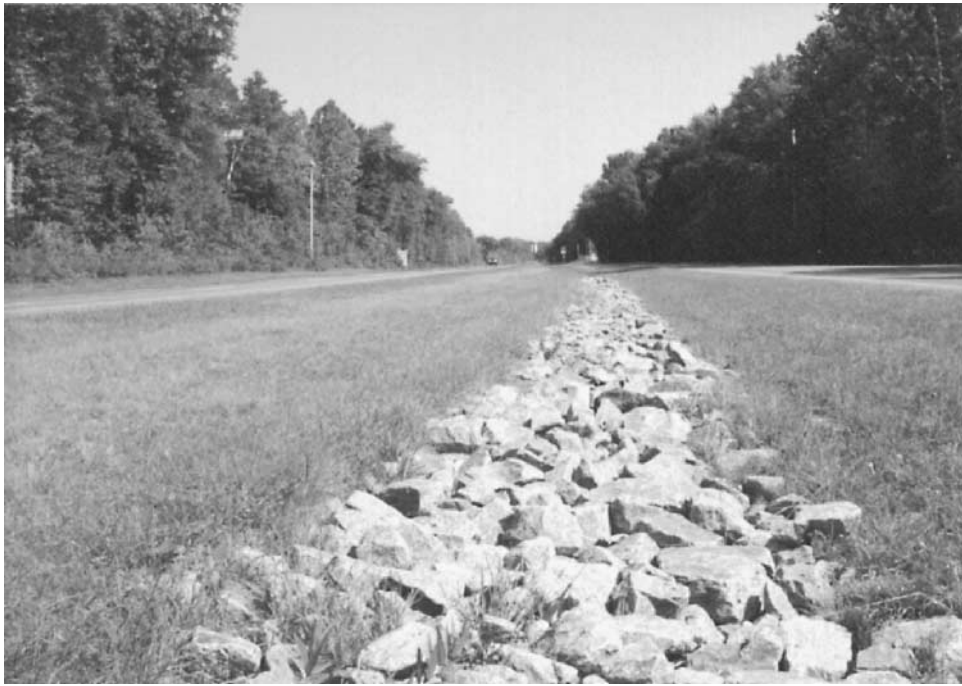
Figure 6.16 Photograph of infiltration trench in median.
