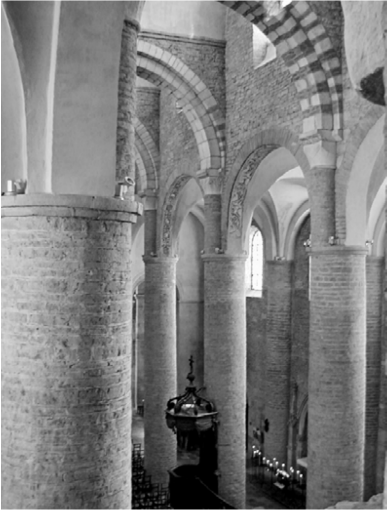
St Philibert, Tournus, early 11th century, nave with its distortions of classical arcades and system of five cross-vaults.
