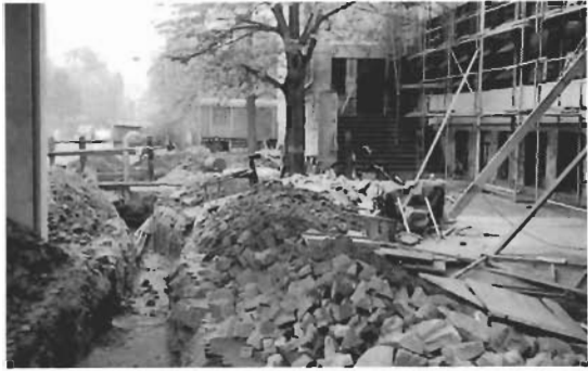
Work at and below ground level, late summer 1976. The BAUHAUS lettering is refitted to the south gable of the workshop wing, October 1976.
