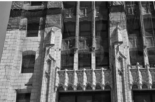
Terra-cotta blocks netted over to prevent from falling to the streets, Mather Tower, Chicago, 1928.
