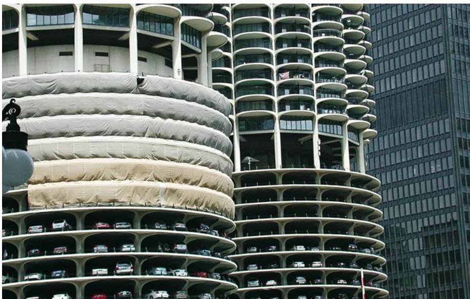
Open concrete balconies are susceptible to reinforcement corrosion caused by weather and de-icing salts. Marina Towers, Chicago.
