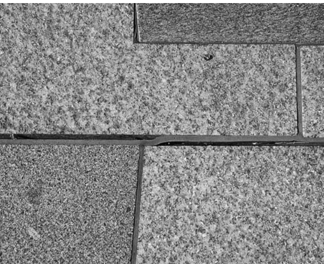
Adhesion failure of sealant on stone.
