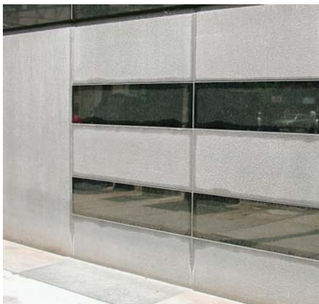
right Stone replacement is the only method for removing the picture-frame effect of sealant joint stains.
