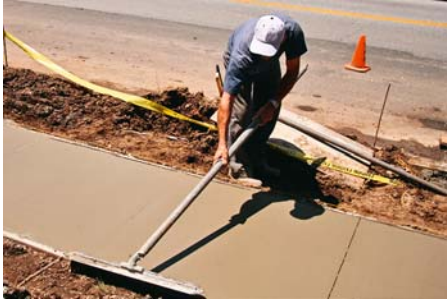
Trowel burn occurs when hard troweling of a concrete surface is executed after the concrete has become too stiff.
