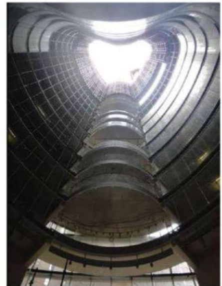
Bligh Street, Sydney: Section through the BIM model, perspective render of the internal atrium and a recent construction photo taken in the atrium. Architect: Architectus + Ingenhoven Architects; builder: Grocon; client: DEXUS Property Group/Cbus Property.
