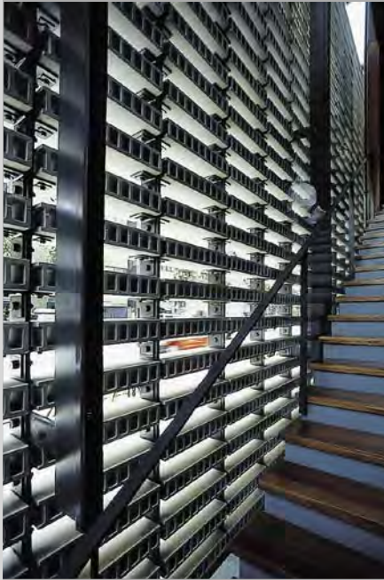
FIG 35. WAKE TOKUYAMA RESTAURANT, DETAIL OF THE EXTERIOR GLASS WALL WITH CONCRETE BLOCK LOUVERS AND INTERIOR STAIRWAY, KENGO KUMA, TOKYO, 2004
