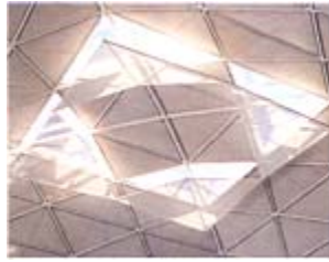
Daylight diffuser below roof light
