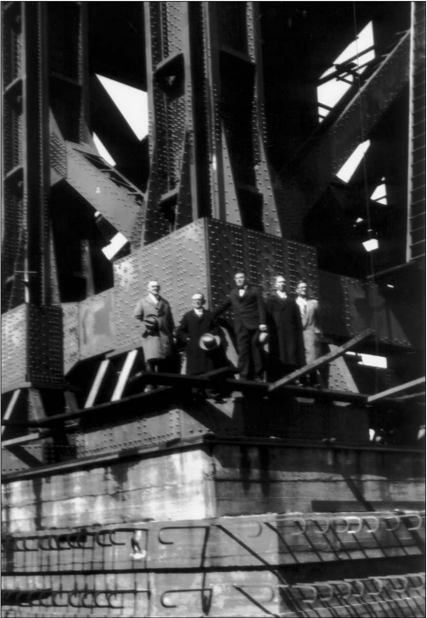
Port Authority engineering staff checking on the mountings of one of the towers. Courtesy of the Local History Department, The Morristown and Morris Township Public Library.
