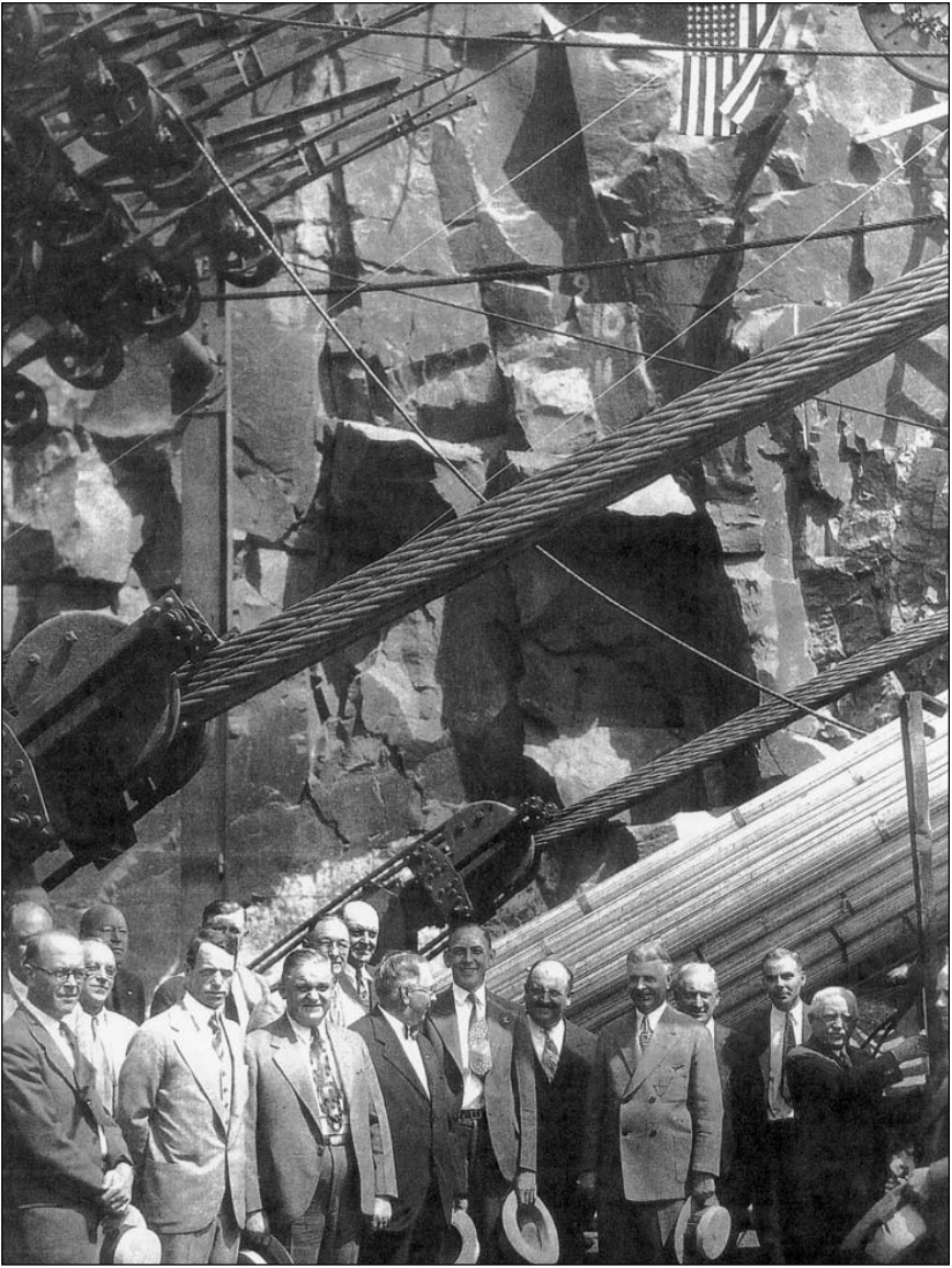
Dignitaries assembled at incomplete New Jersey anchorage carved into the Palisades. Othmar Ammann is in first row, second from left. John F. Galvin, Port Authority chairman, is about to push the button sending the last of 105,684 barrel cable wires spinning across the river. Courtesy of Dr. Margot Ammann Durrer.
