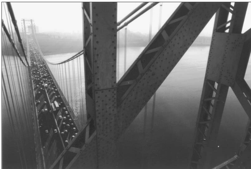
The world from on high in one of the towers. Courtesy of the Port Authority.
