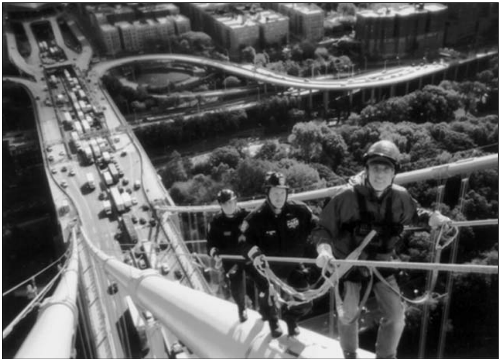
Photo of the author scaling barrel cable C toward the New York tower with Sergeant Kevin Cottrell and Lieutenant Richard Munnely of the Emergency Service Unit Police immediately behind him.
