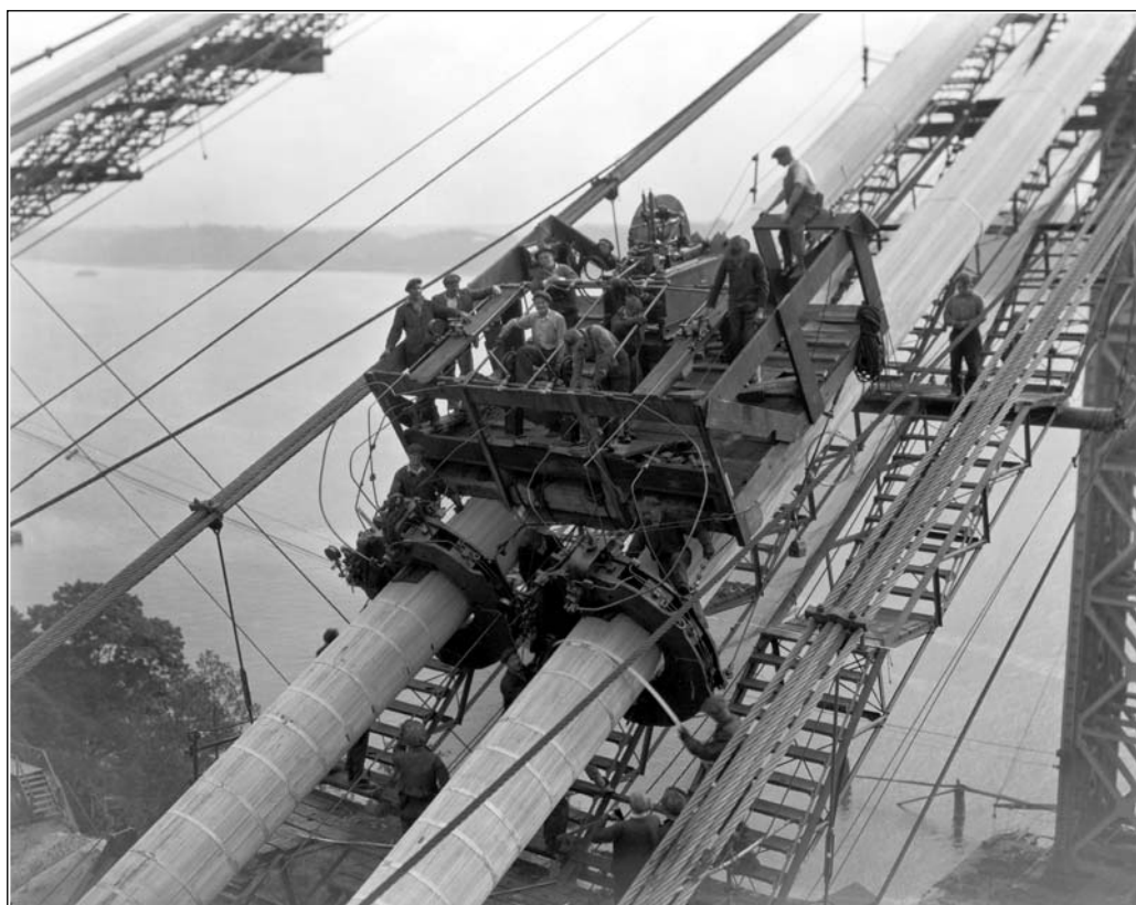
Men operating the squeezer, which is simultaneously compressing the components of two barrel cables into a rounded form. Courtesy of the Port Authority.
