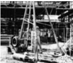
The drilling rig at the BRE environment building, used to drive a 70m deep borehole into a chalk aquifer
