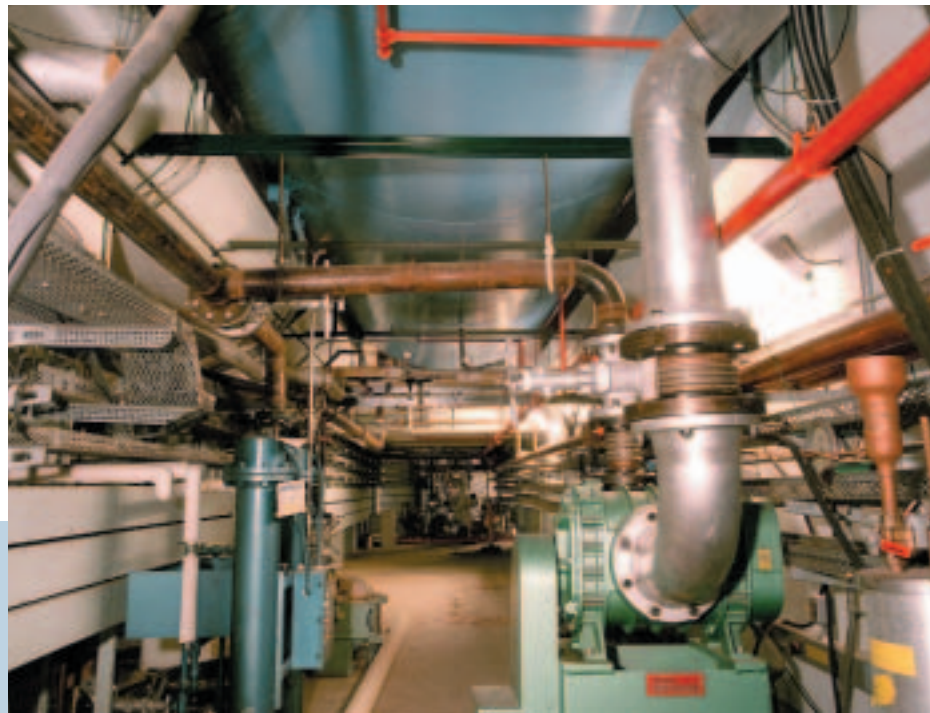
The LANL Ion Beam Facility mechanical room.
