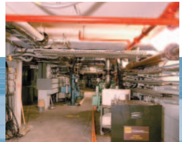
The LANL Ion Beam Facility mechanical room.
