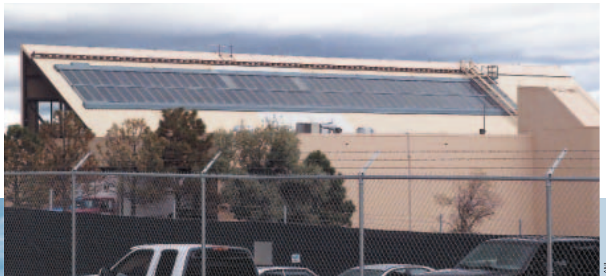
Solar hot water system on the LANL Otowi Building. The excellent solar resources in Los Alamos make solar hot water systems a viable solution for meeting DHW loads and preheating water for process and space heating loads. These systems have a high first cost, but very low operating costs. A year-round water heating load, such as for cafeteria, locker room facilities, and process loads, is required to make solar hot water systems cost-effective.
