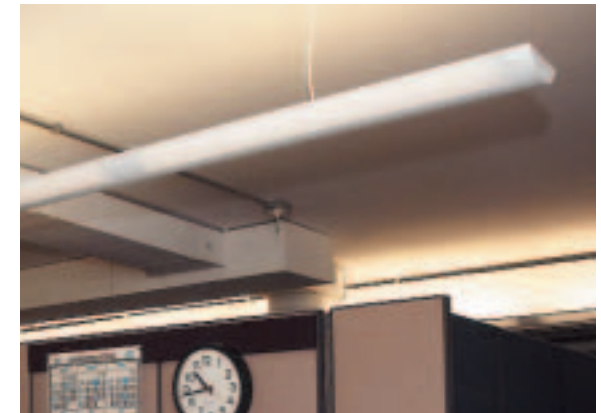
Indirect lighting fixtures with T-5 lamps in the LANL PM Division offices reduces glare and provides more uniform ambient light.
