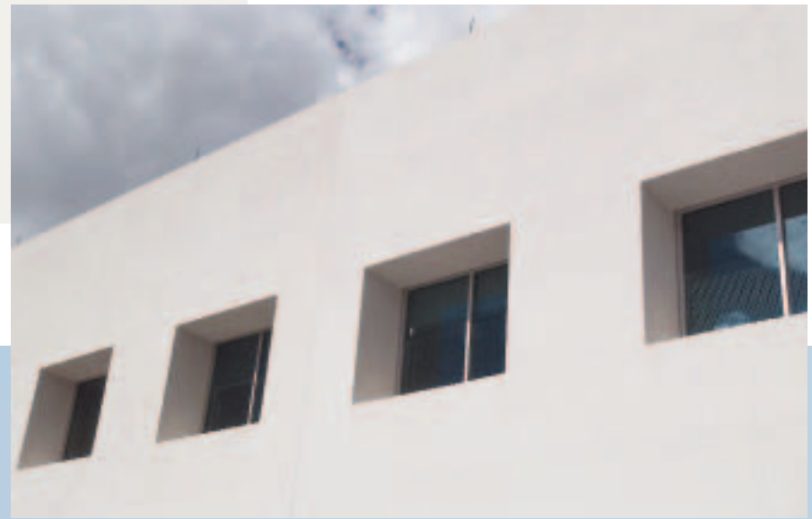
Placing the windows deep in the south-facing wall helps to shade the window to minimize direct solar gains and reduce perimeter cooling loads.
