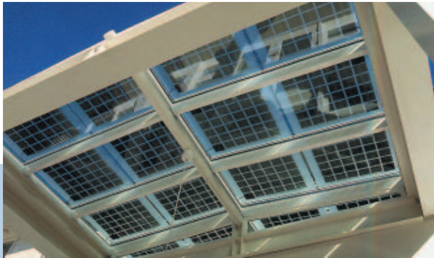
The skylighted entryway at the Thoreau Center for Sustainability at Presidio National Park, San Francisco, California, uses photovoltaic cells that are laminated to the skylight glass to produce electricity as well as to shade and daylight.
