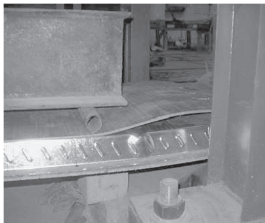
Figure 12. Buckling of profiled steel sheet in midspan.
