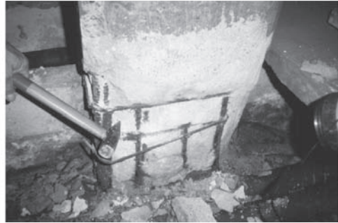
(b) Steel reinforcement after 10 years in closed area
