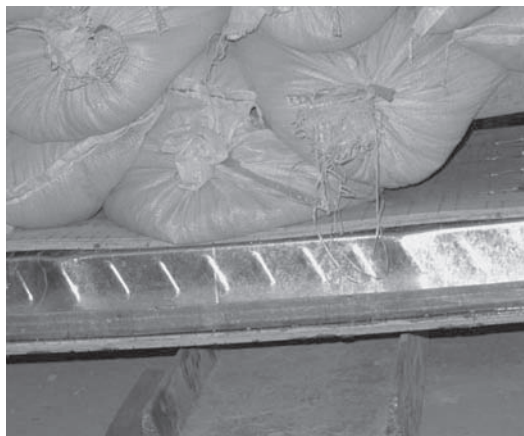
Figure 10. Buckling of profiled steel sheet.
