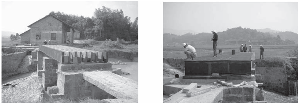
Figure 4. Construction stages: (a) installation of bamboo girders; (b) installation of water proof materials.
