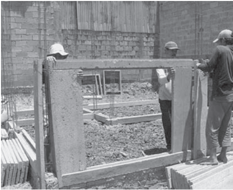
Figure 14. The assembling of prefabricated partition wall panel in accordance with middle beam.
