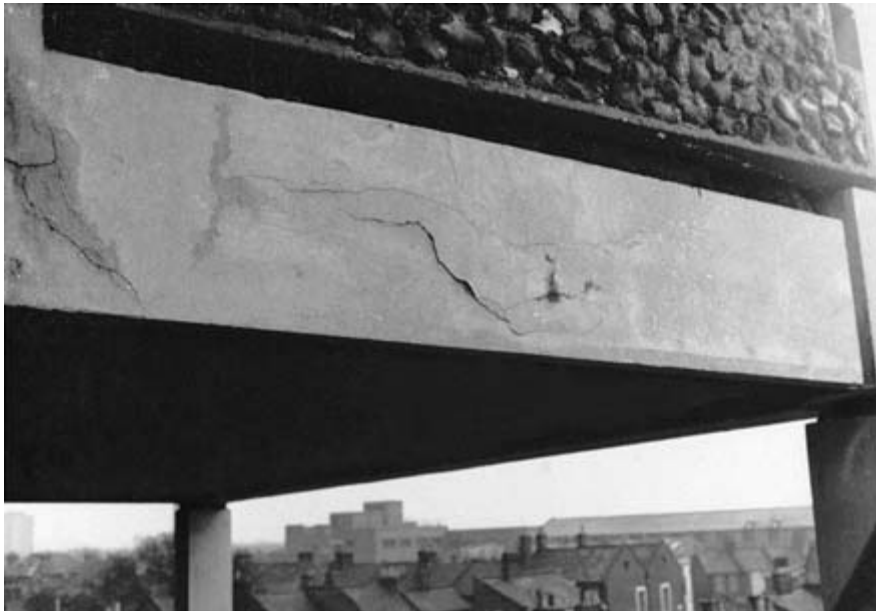
Figure 7.2 Corrosion of reinforcement causing cracking of concrete (courtesy of SGB Group Publicity).
