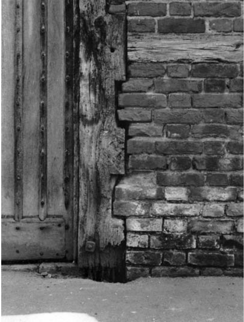
Figure 8.3 Effects of rising damp and woodworm in a timber framed building.
