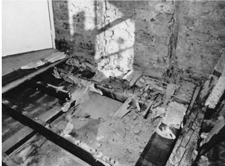
Figure 9.1 Dry rot spore dust in floor joists and partition (courtesy of SGB Group Publicity).
