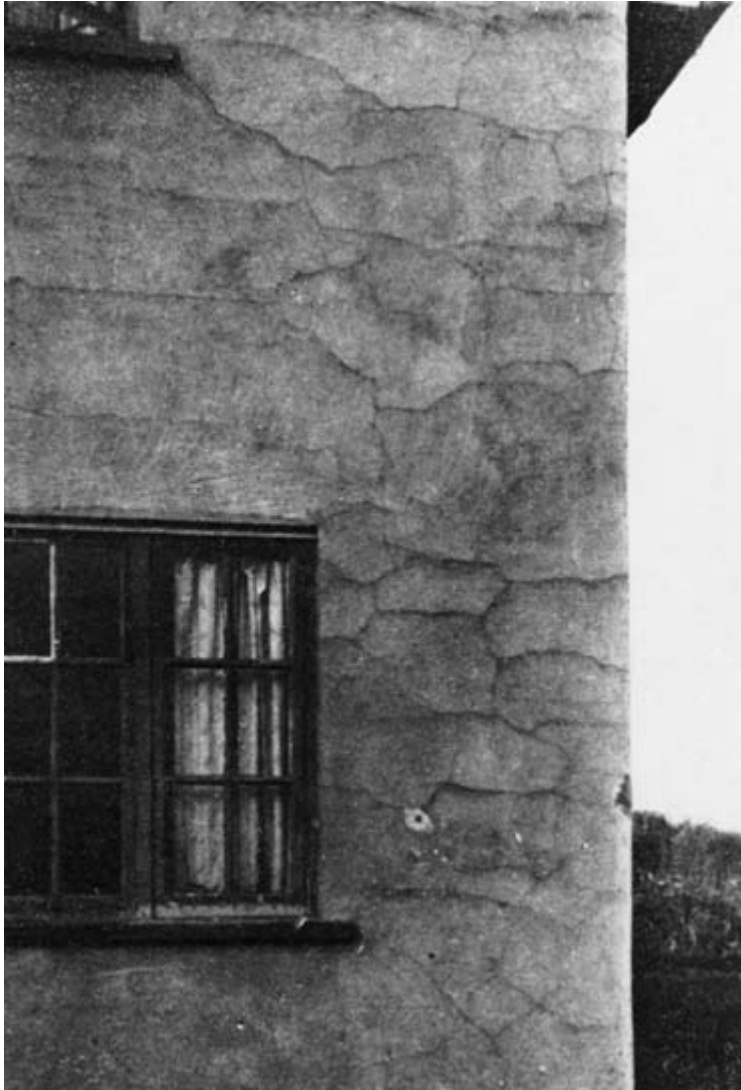
Figure 13.1 Cracked rendering as a result of sulphate action.
