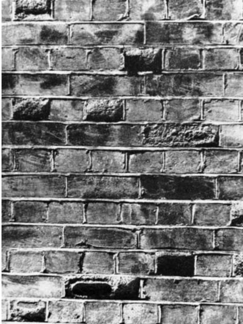
Figure 6.8 Surface decay of brickwork due to crystallisation of salts.
