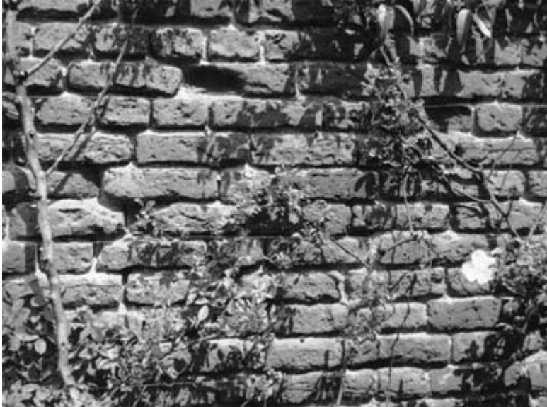
Figure 6.14 A fairly common defect caused by shrubs sending their roots into brick joints.
