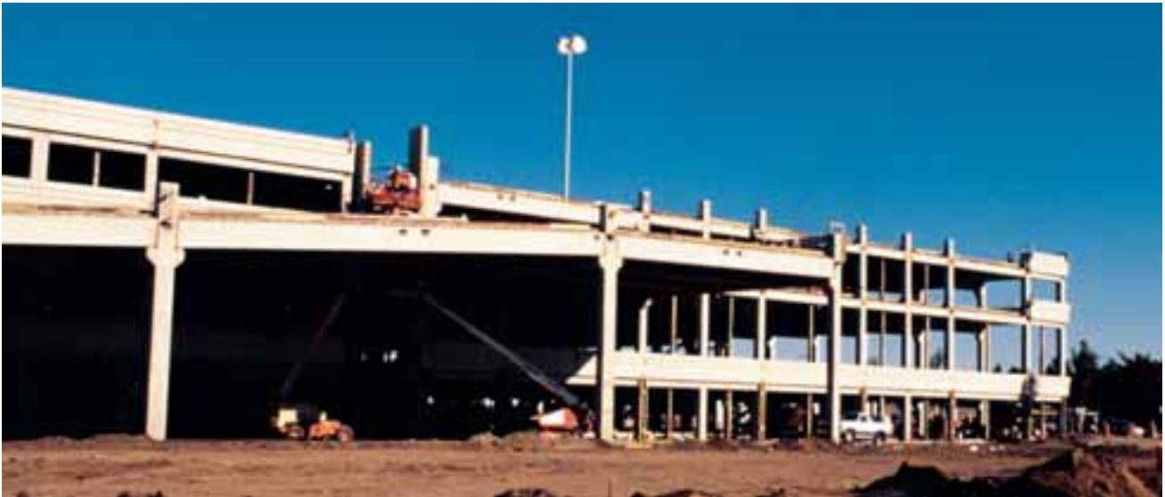
The new framing design helps the Roosevelt Field Mall parking structure resist wind loads, as there are no special seismic needs required in this region. It also met the owner's desire for open spans unobstructed by conventional shear walls. The project was part of a $150-million capital-improvement program at the mall.
