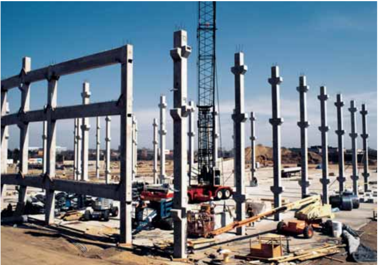
Several advantages are offered by the hybrid system, which combines standard reinforcing steel with high-strength, post-tensioning steel cables to provide both inelastic flex to absorb energy and elastic action to offer shear and moment resistance. The benefits include long-term cost efficiencies, simplicity of design, speed of erection and safety enhancements.
