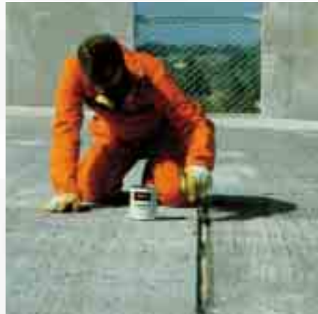
Joint sealants should be periodically inspected and replaced if necessary.
