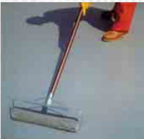
Polyurethane, epoxy and other surface sealers should be reapplied every 3 to 5 years.
