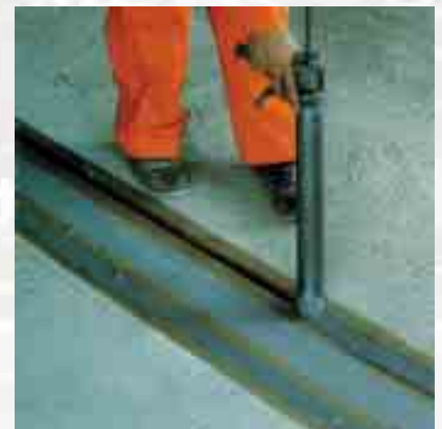
Expansion joints may require recaulking.
