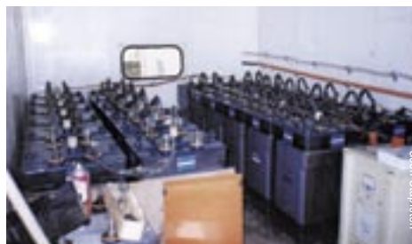
A battery bank
