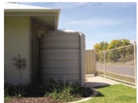
The 2 kL rainwater tank at the S/E corner
