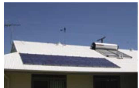
Two arrays of PV cells and the solar H/W unit
